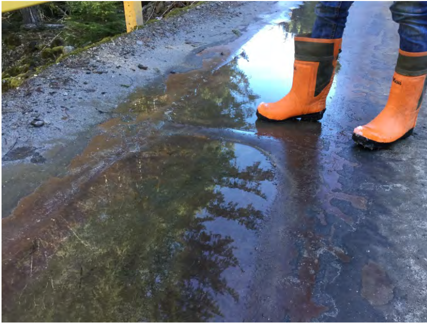
Deck plate deformation noted on wheel path
